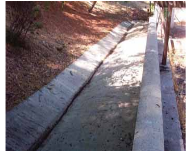
Above: Portion of a drainage ditch along the southern boundary of the project site.
