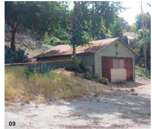
09 GARAGE/STORAGE SHED (YEAR UNKNOWN)
